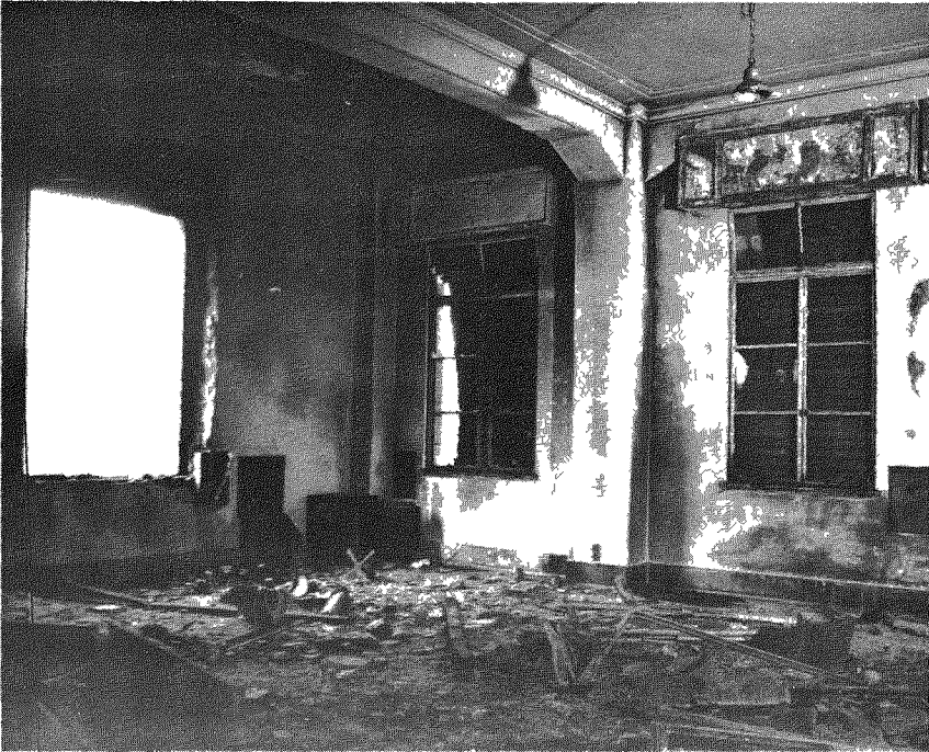
Figure 7.95. Fire shutters in building blown in or damaged by the blast; shutter at center probably blown outward by blast passing through building (0.57 mile from ground zero at Hiroshima).
